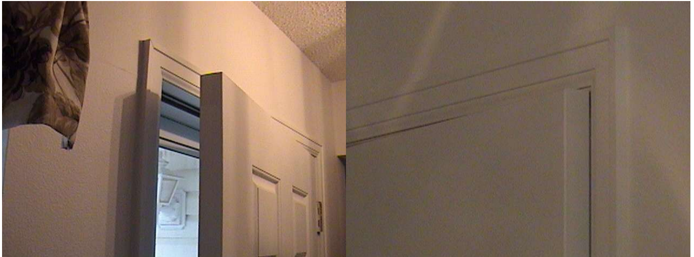
Repair: Miss aligned door(s) stick or do not close, the door(s) should be adjusted to work properly.
